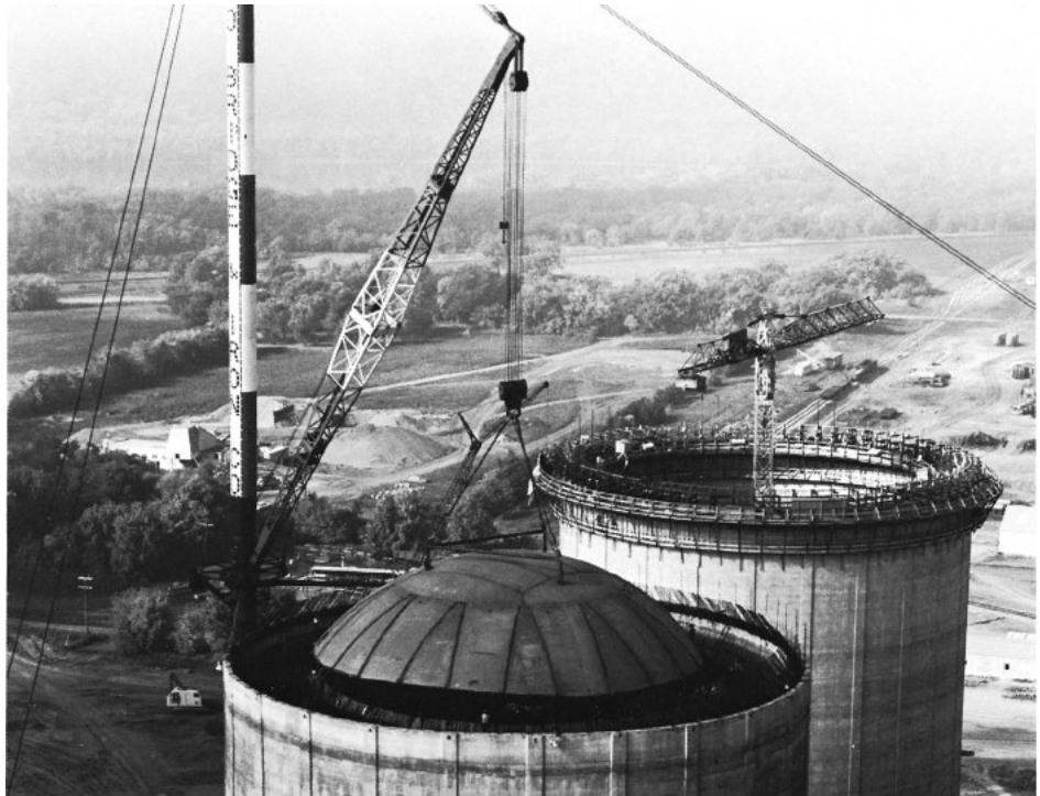
FIGURE 2.75 (Photo courtesy of CBI Industries Inc.)
