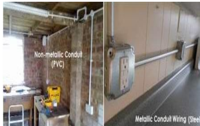
Fig.2.8. Surface conduit wiring.
