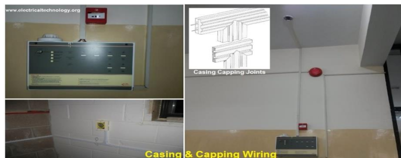
Fig.2.5. Wooden casing and capping wiring.
