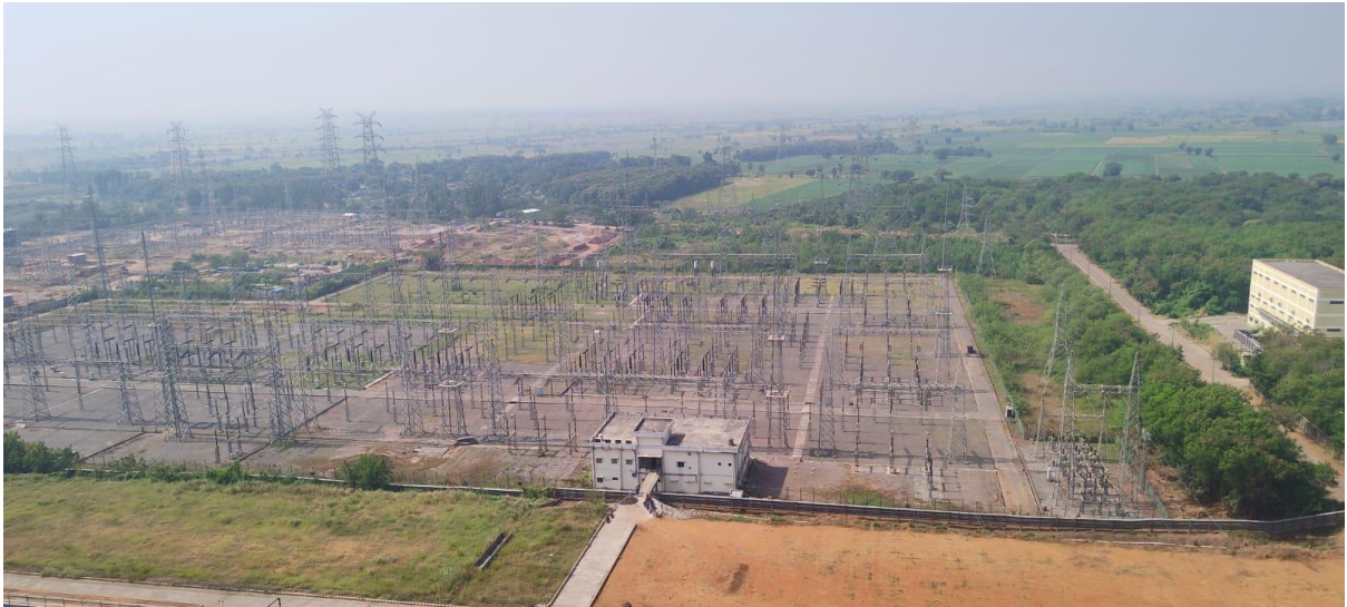
21/400 KVA STEP UP TRANSFORMER
